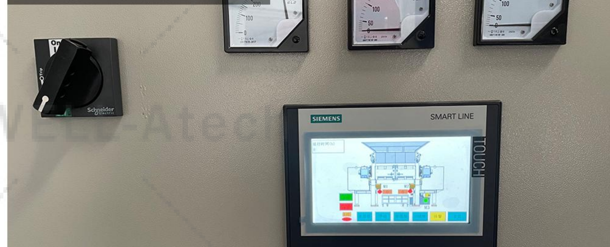
电控 Electrical Control
